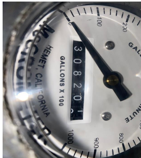
Finish discharging at 03:14, 02-03-2024
