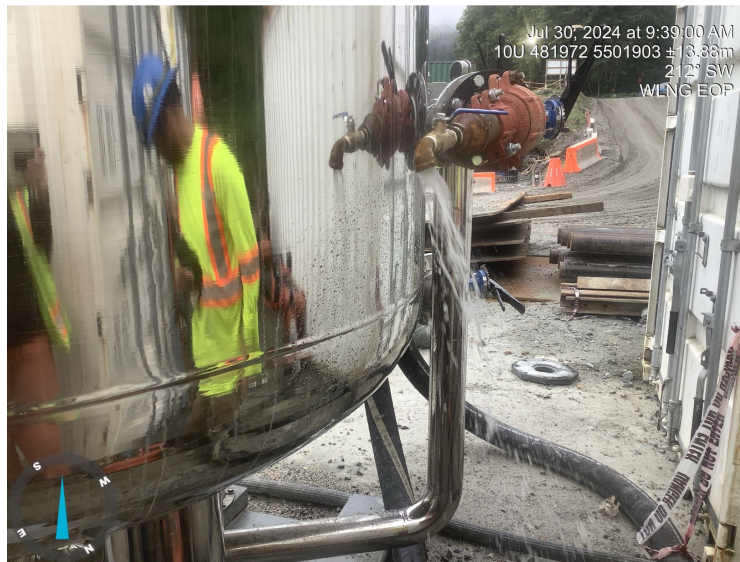
Photo: 1 Location: WLNG EOP Description: Spigot at holding tank
