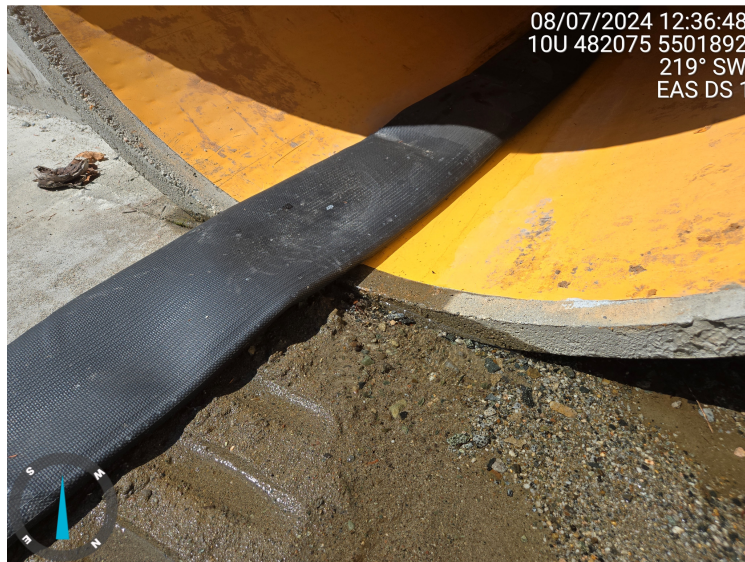
Photo: 1 Location: EAS DS 1 - original Description: Low flow in culvert
