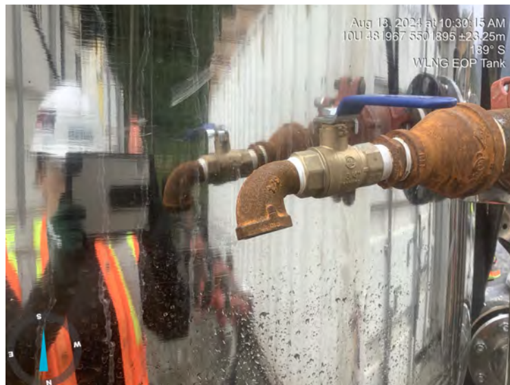
Photo: 2 Location: WLNG EOP TANK Description: Spout connected to tank
