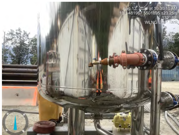
Photo: 1 Location: WLNG EOP TANK Description: Tank containing treated water
