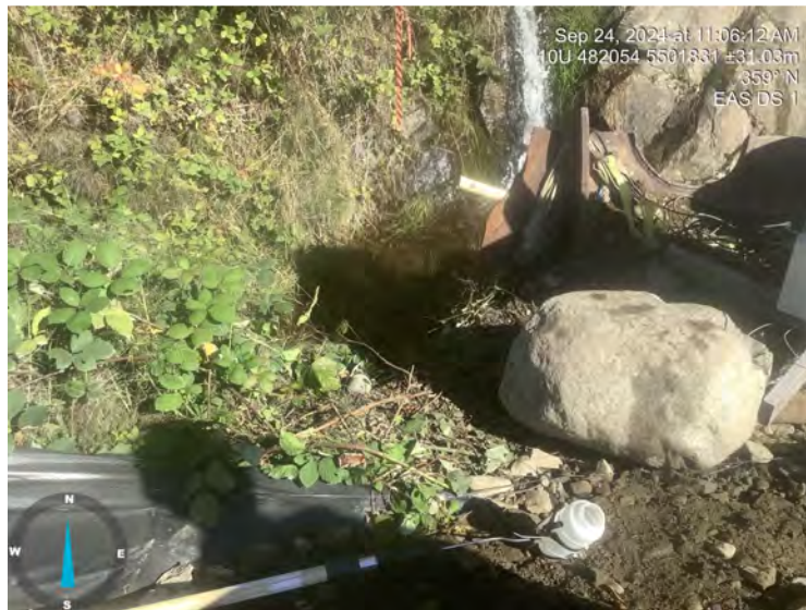
Photo: 5 Location: EAS DS 1 Description: Poorly implemented sediment fence next to East Creek
