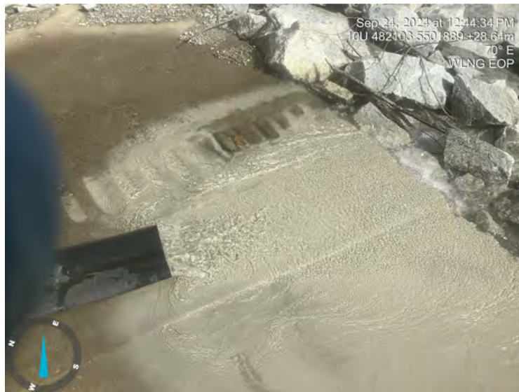
Photo: 5 Location: WLNG EOP Description: Fan of sediment at discharge pipe.
