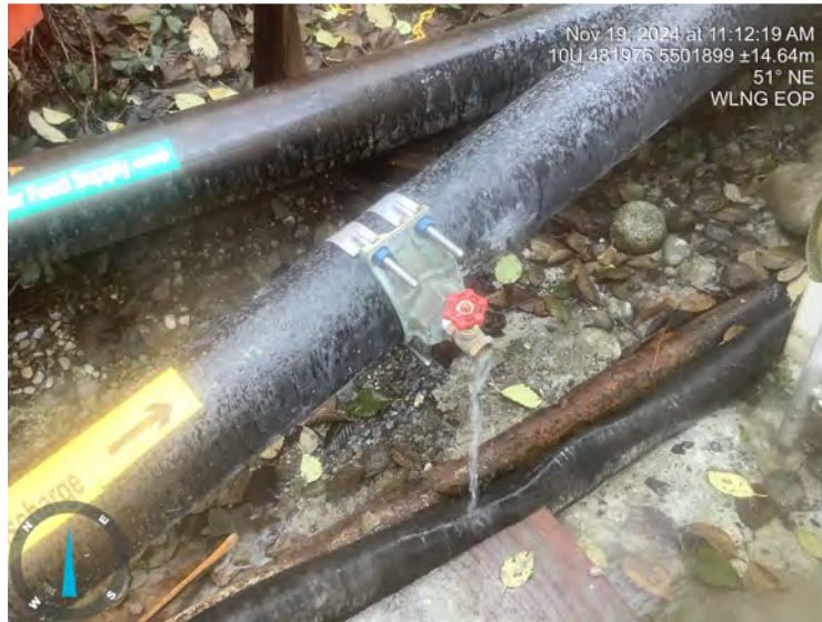
Photo: 1 Location: WLNG EOP Description: Discharge sampling point
