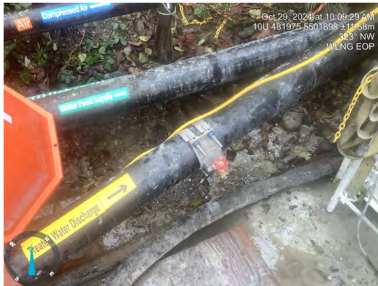
Photo: 1 Location: WLNG EOP Description: Spigot in discharge hose.
