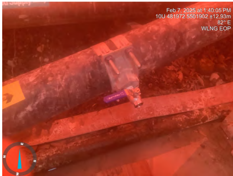
Photo: 1 Location: WLNG EOP Description: Spigot off
