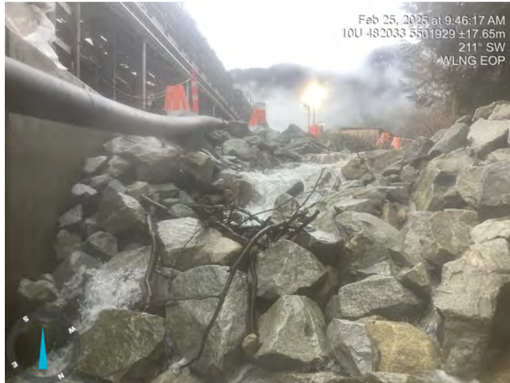
Photo: 2 Location: WLNG EOP Description: Pipe source of treated water
