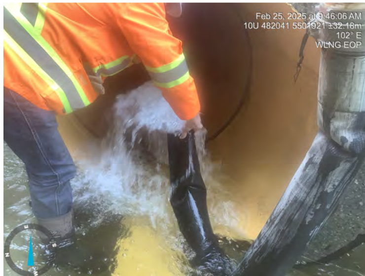
Photo: 1 Location: WLNG EOP Description: End of the pipe hose
