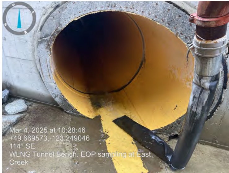
Photo: 1 Location: WLNG EOP Description: End of pipe collection
