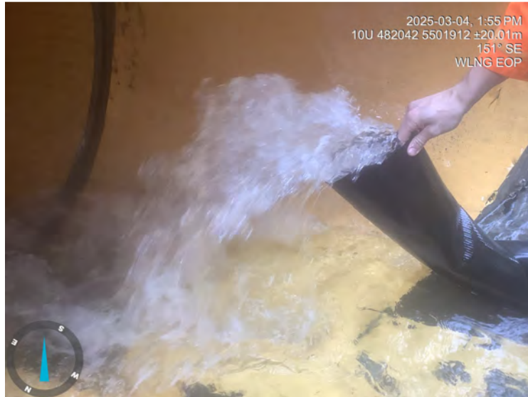
Photo: 4 Location: WLNG EOP Description: EOP discharging
