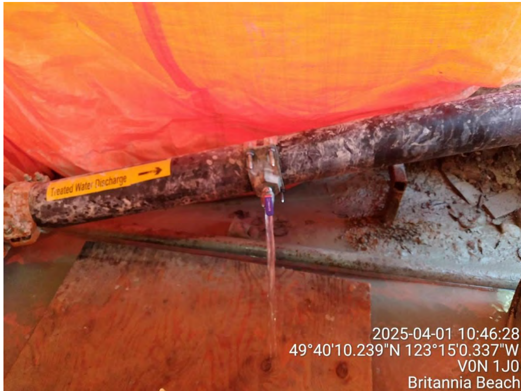
Figure 1 WLNG End of pipe sampling.
