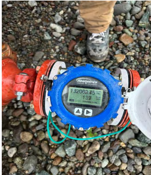
Photo 1: Discharged flow meter (beginning of discharging), November 14 th
